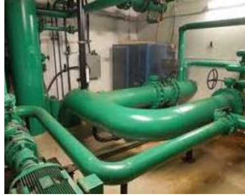
OTs chilled water supplies routed through main pump
