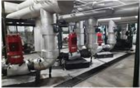
Optimized usage of primary pumps in HVAC chiller system
