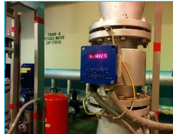
System level Water Metering facility
