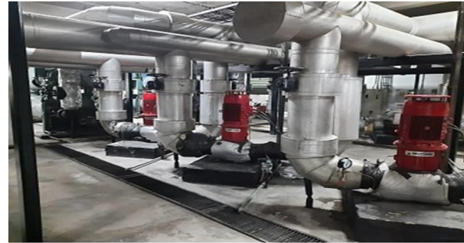
Condenser Pumps with VFD
