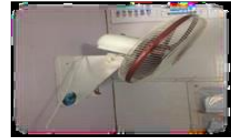
Damaged pedestal fan converted into wall mounted fan in engineering Area
