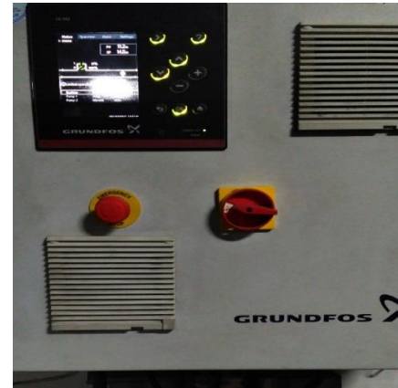
VFD operated AHU's
